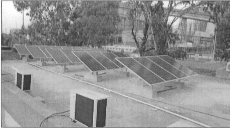
Solar PV Plant in Canteen.
