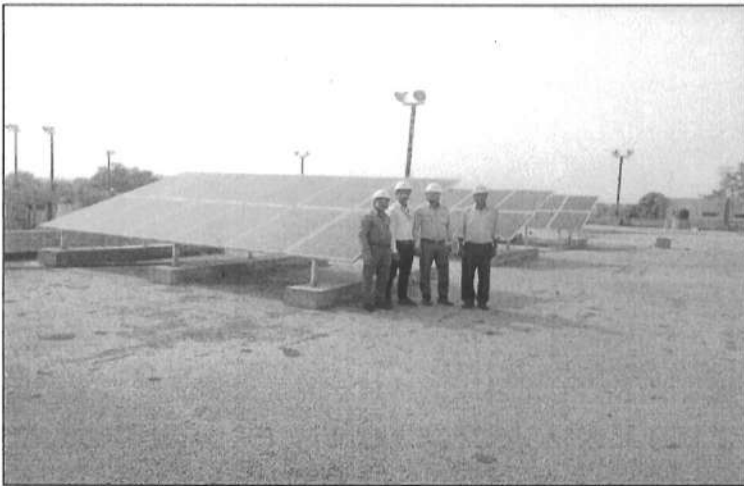
Solar PV Plant in DM Plant.
