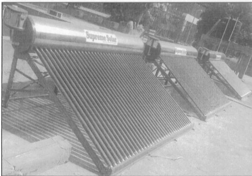
Solar Water Heater at Plant
